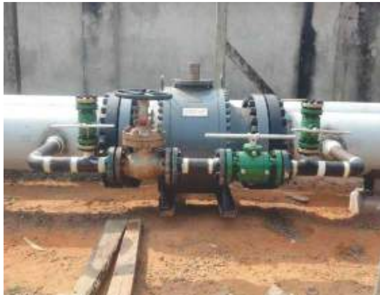
Refurbished 10" pig launcher/receiver
